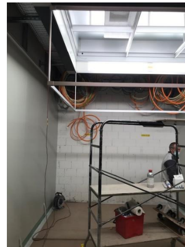
Installationen in OP-Saal OG01
